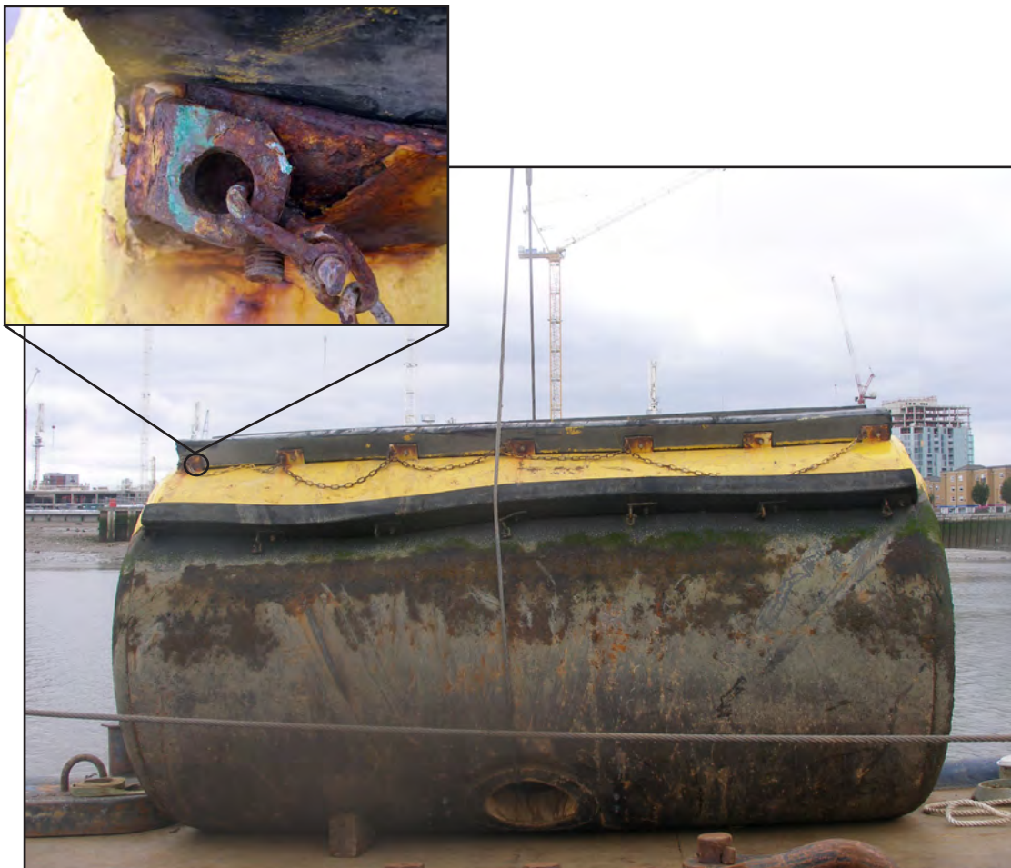
Figure 24: Contact buoy - fender support lug damage and (inset) evidence of paint from barge
