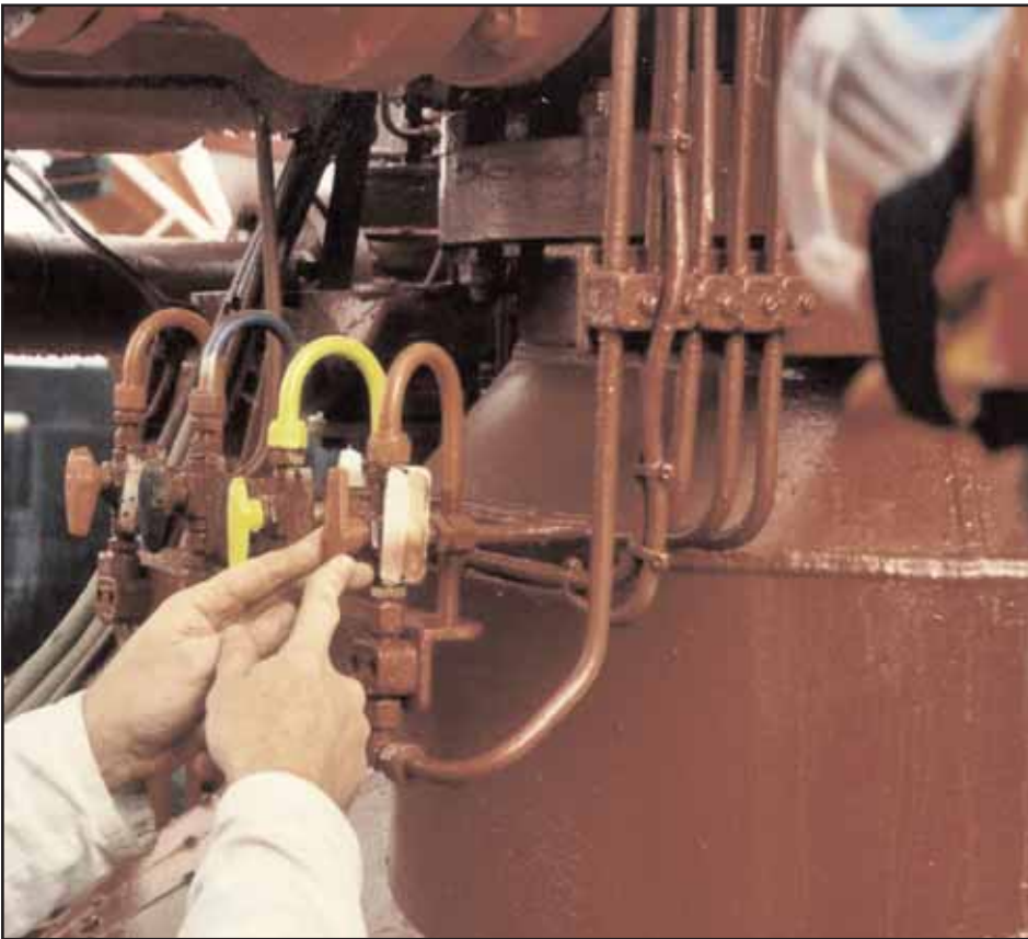
Forward tank pneumatic valve controls
