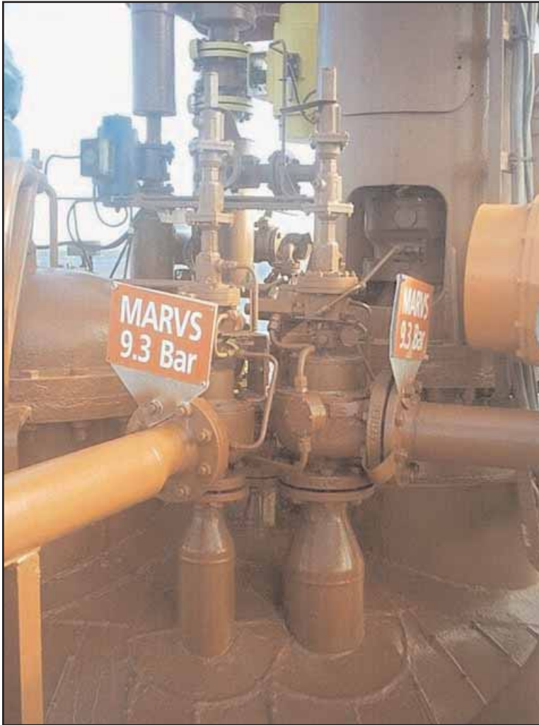
Forward cargo tank pressure vacuum valves
