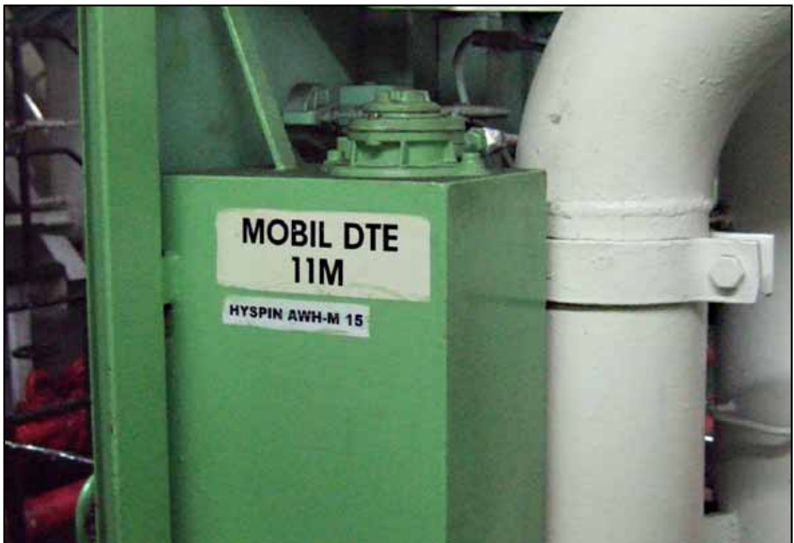
Hydraulic storage tank
