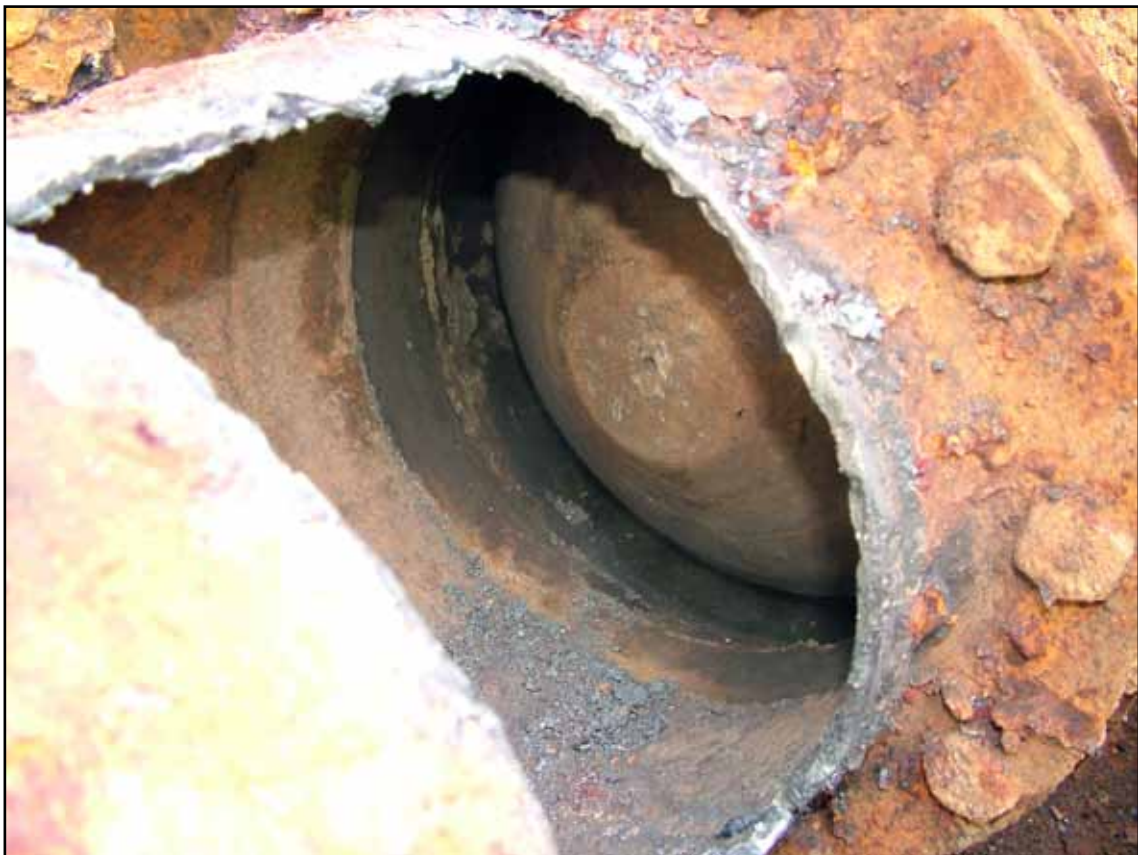
Port non return valve not sealed
