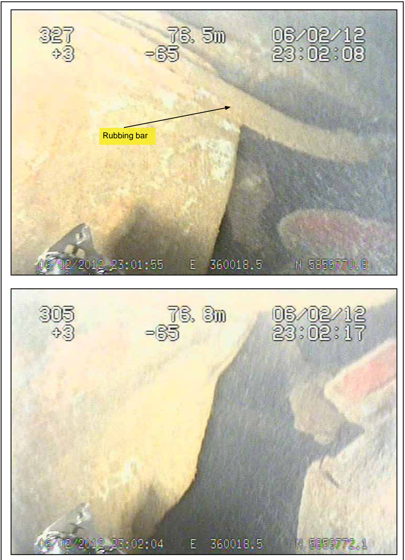
Figures 70a and 70b: Stills from ROV footage showing signs of brittle failure in the lower structure in way of the main fracture path
