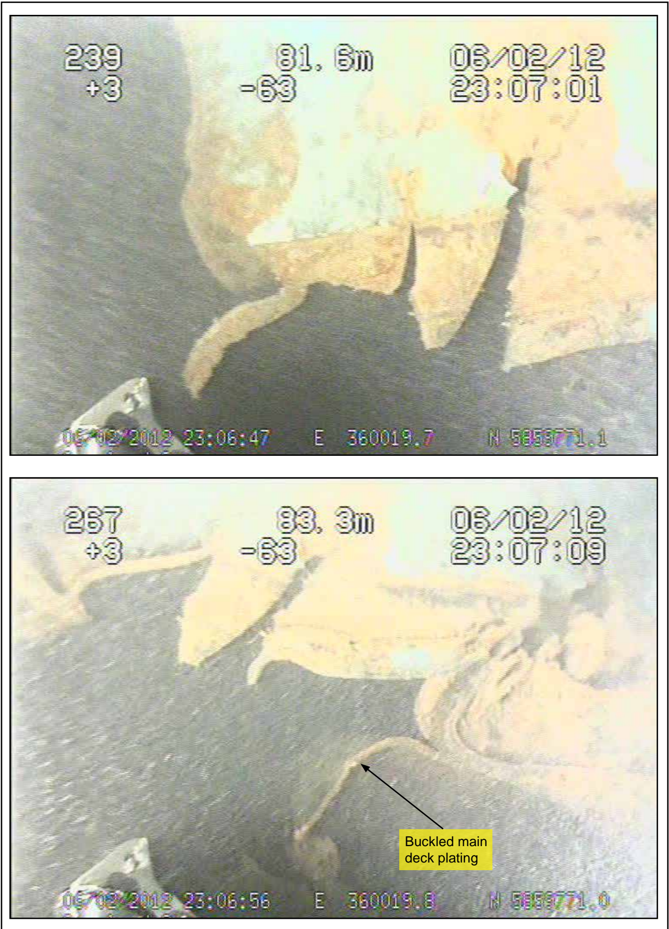
Figures 69a and 69b: Stills from ROV footage showing signs of ductile failure in the upper structure in way of the main fracture path
