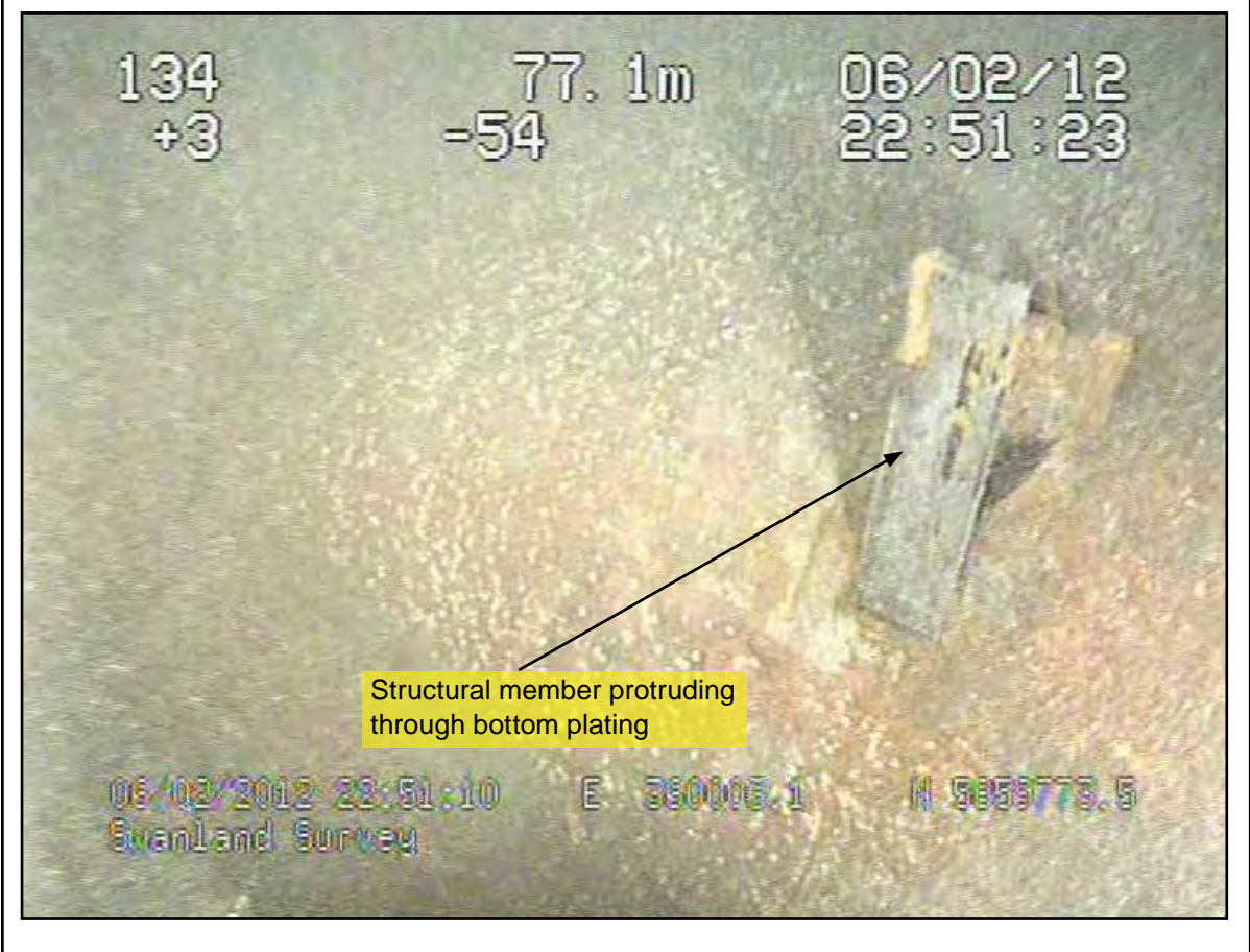
Figures 27a and 27b: Stills from ROV footage showing structural members protruding through Swanland's bottom plating
