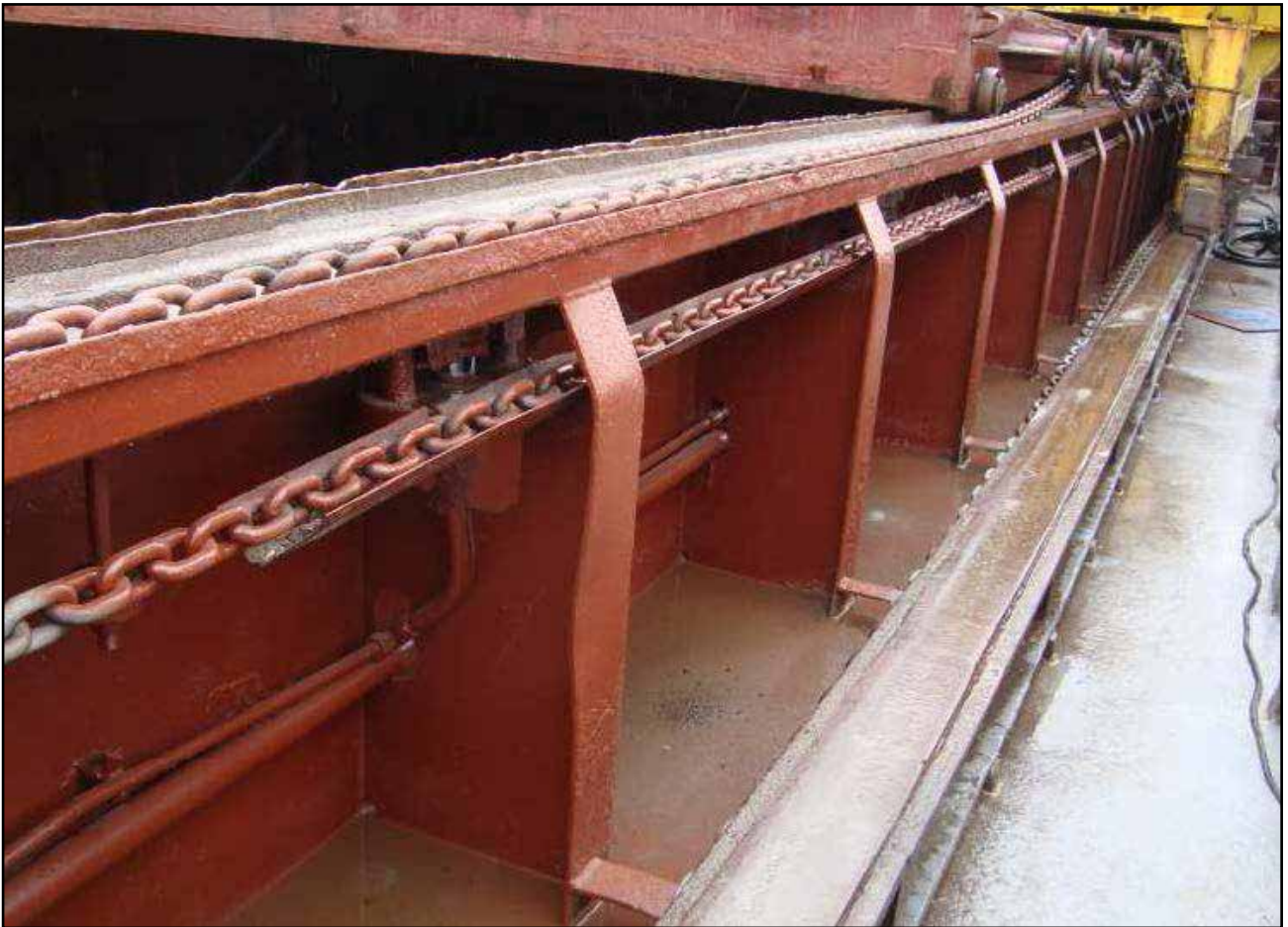
Figures 39a and 39b: Water trap area between excavator carriage rail and cargo hold hatch coaming on Swanland
