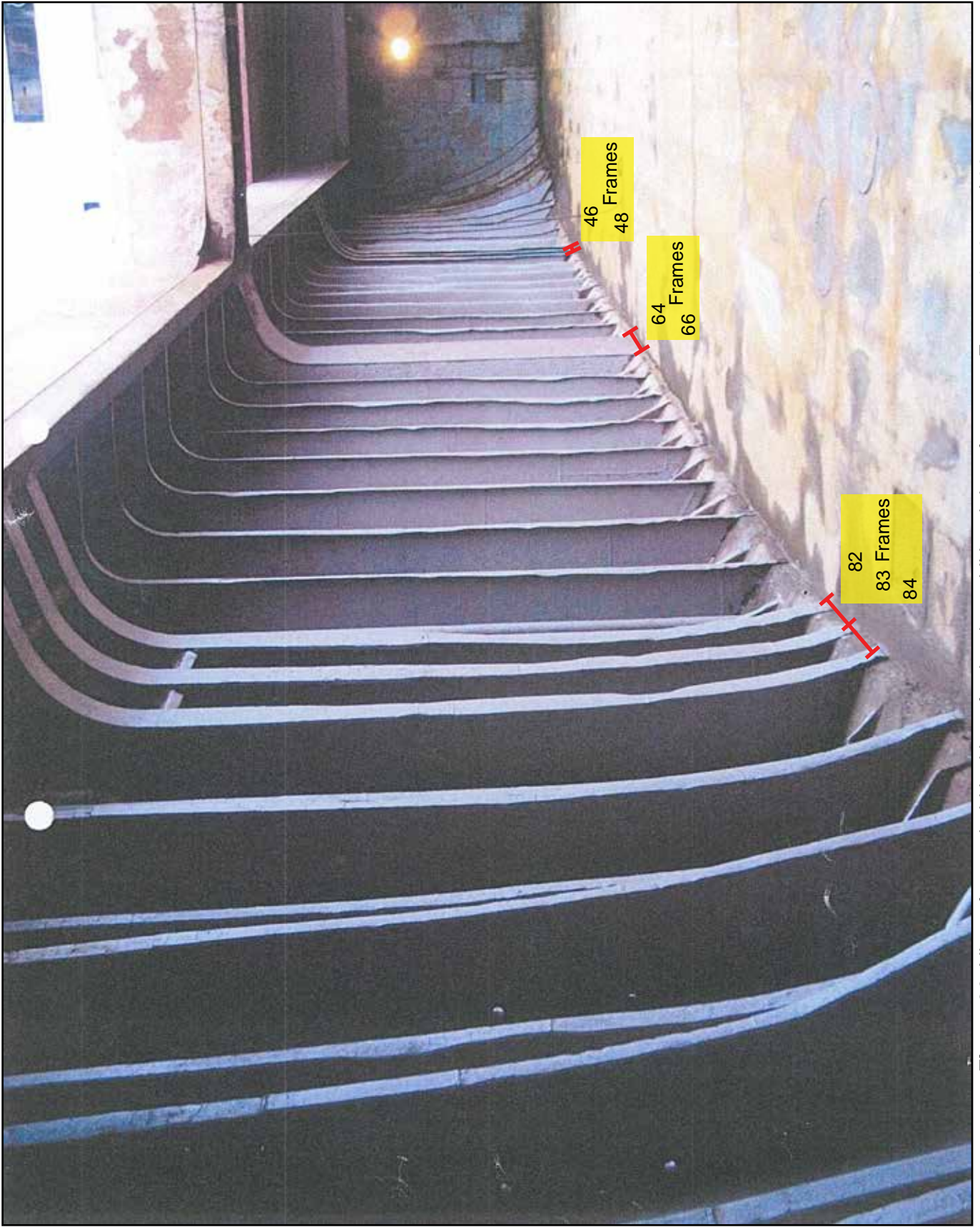
Figure 36: View of cargo hold looking aft, showing additional deep frames at Frames 47, 65 and 83
