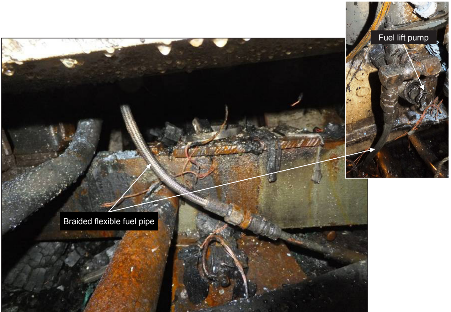
Figure 3: Auxiliary engine braided flexible fuel pipe
