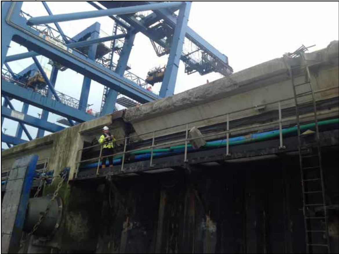
Figure 5: Damage to quay, Northfleet Hope Container Terminal
