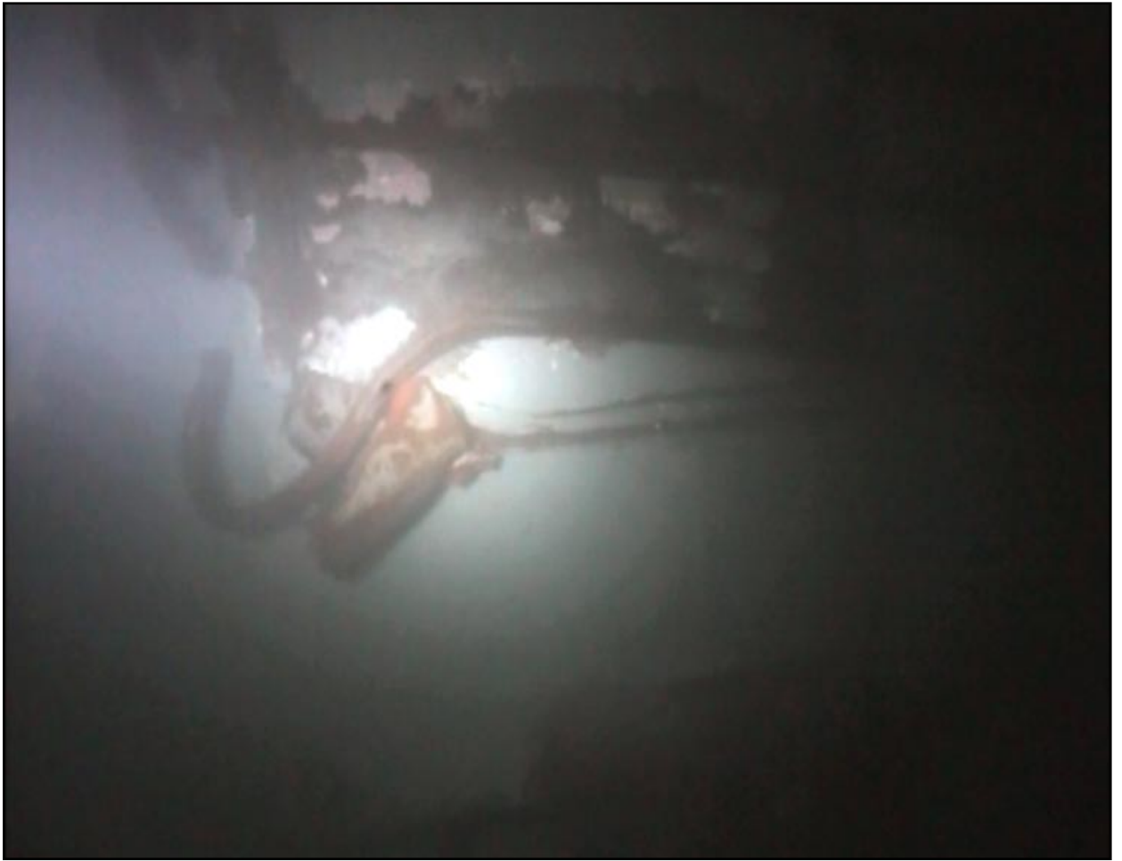
Damage to sea valve protection cage
