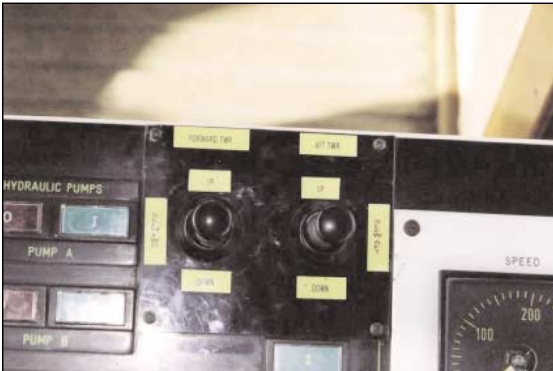
View of loading tower controls
