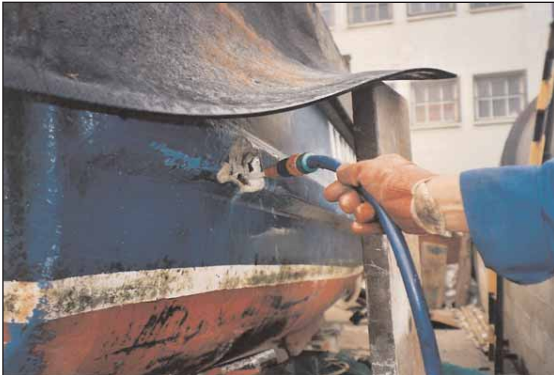
Hose test on damage
