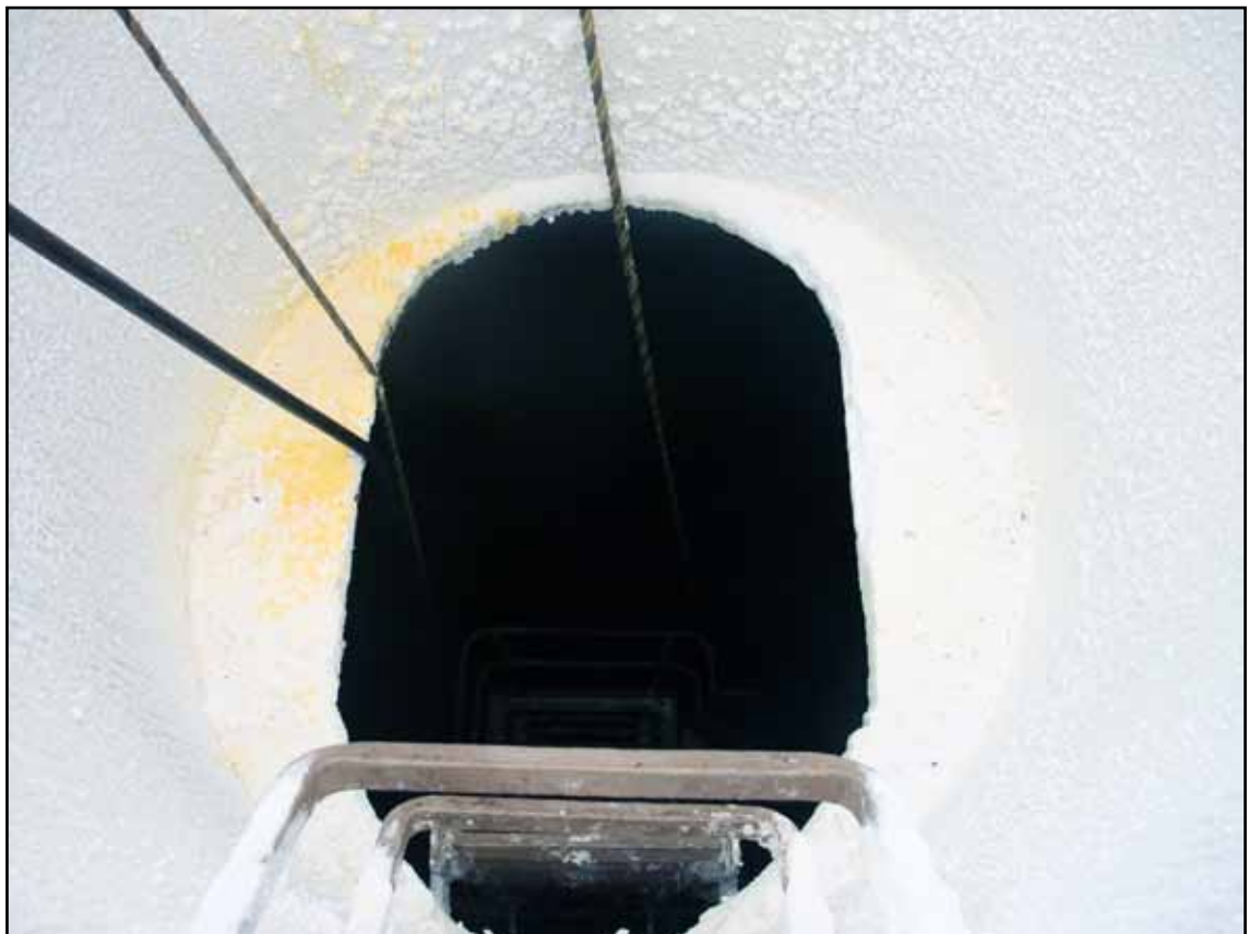
No 2 cargo tank hatch coaming showing solidified stearin coating
