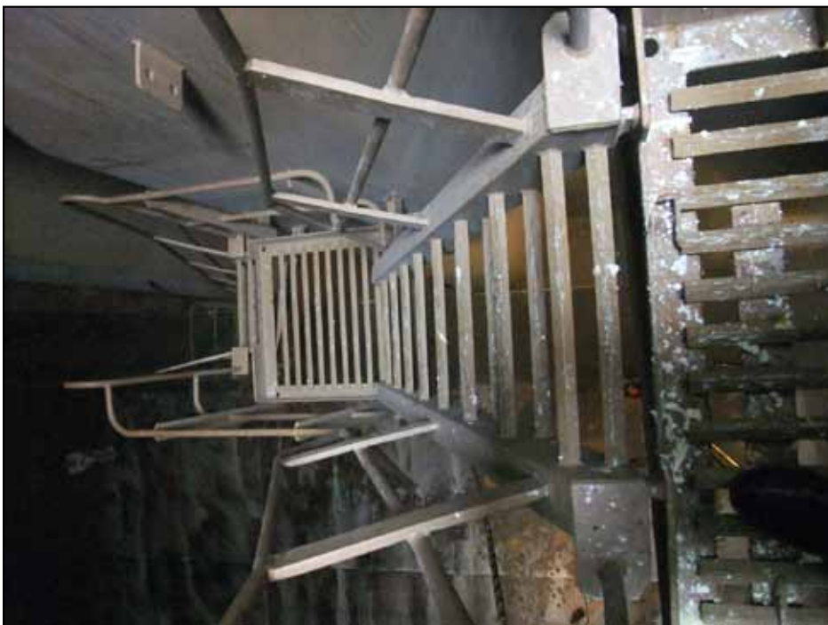
No 2 cargo tank - angled ladders
