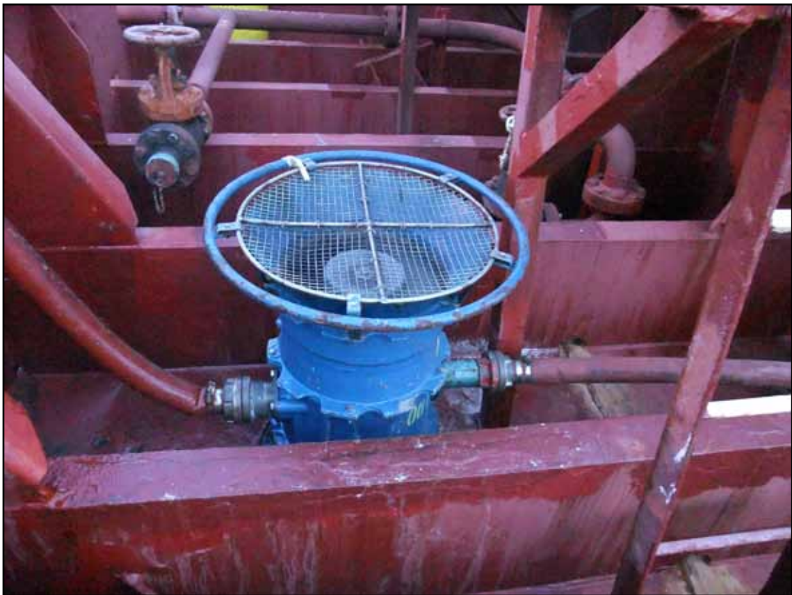
Water-driven forced ventilation fan
