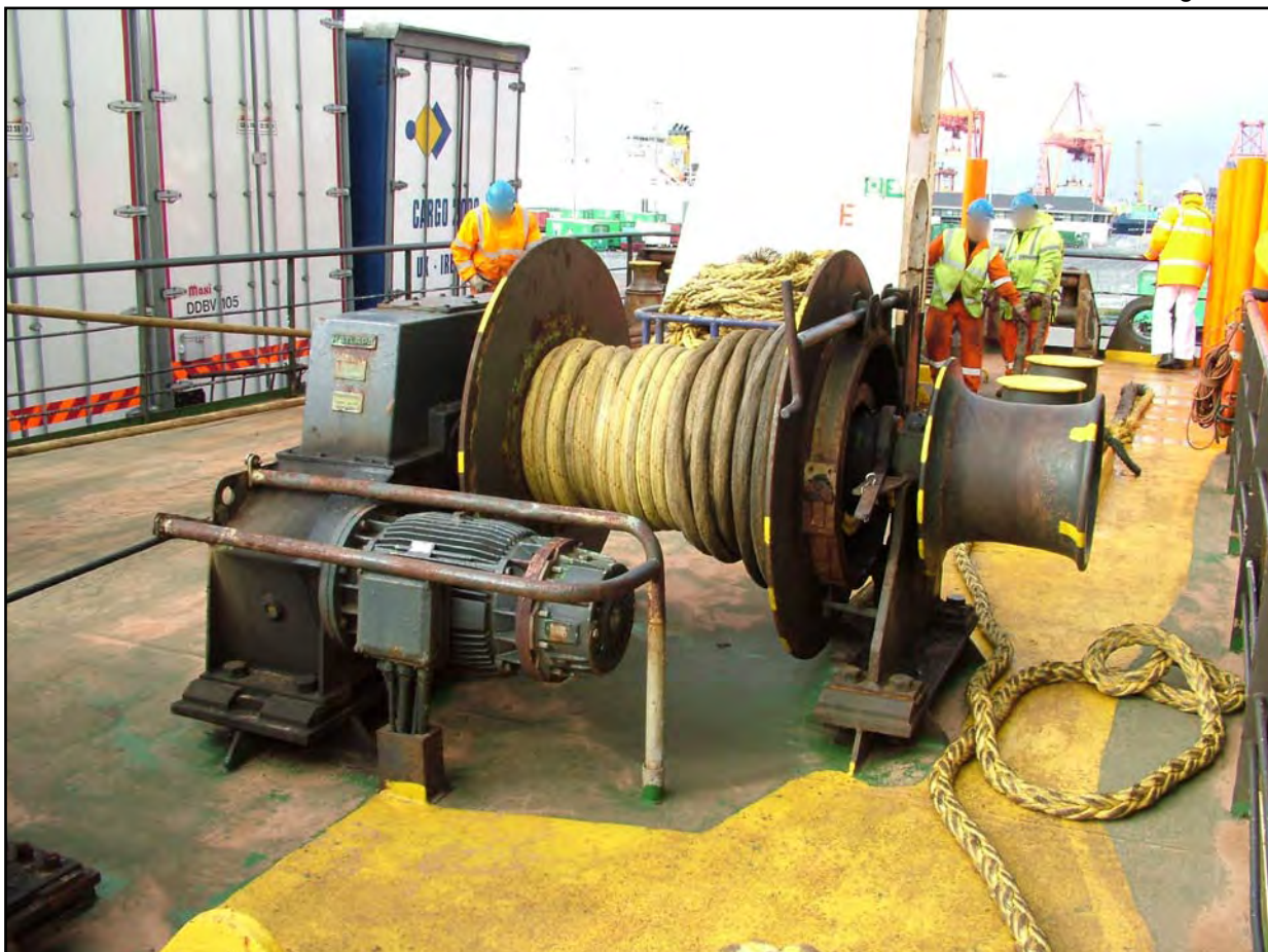
Orientation of band brake on mooring winch
