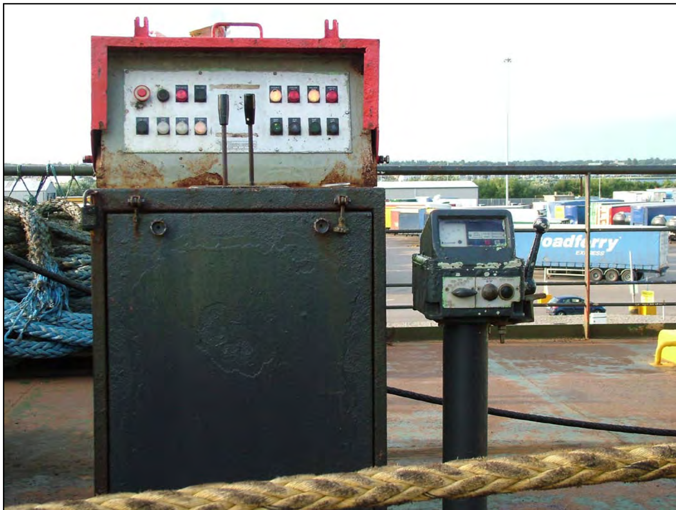
Stern line and stern ramp winch controls
