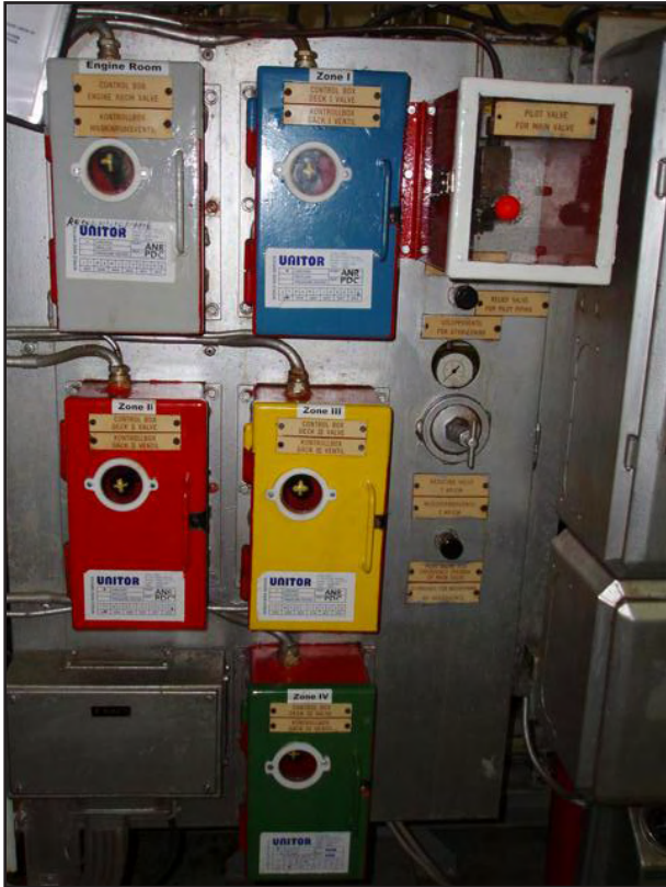
Colour coding of distribution valves and protective enclosure to main release valve on CO 2 room control panel
