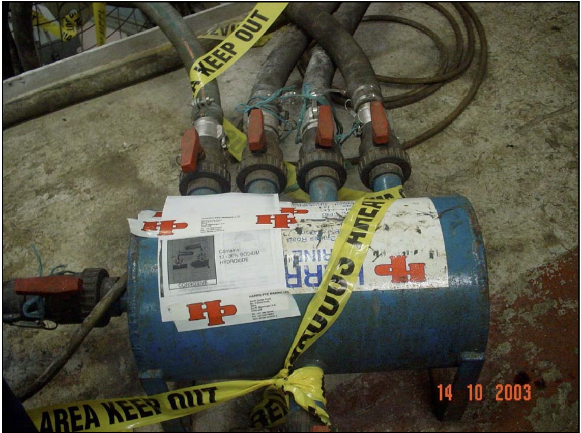
Manifold and connecting hoses
