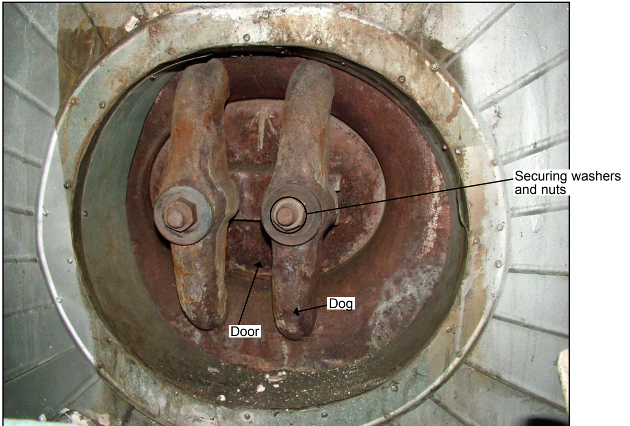
Starboard boiler steam drum, door arrangement
