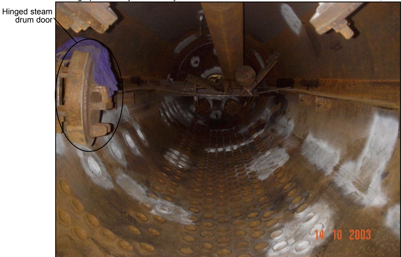
Starboard boiler – open steam drum
