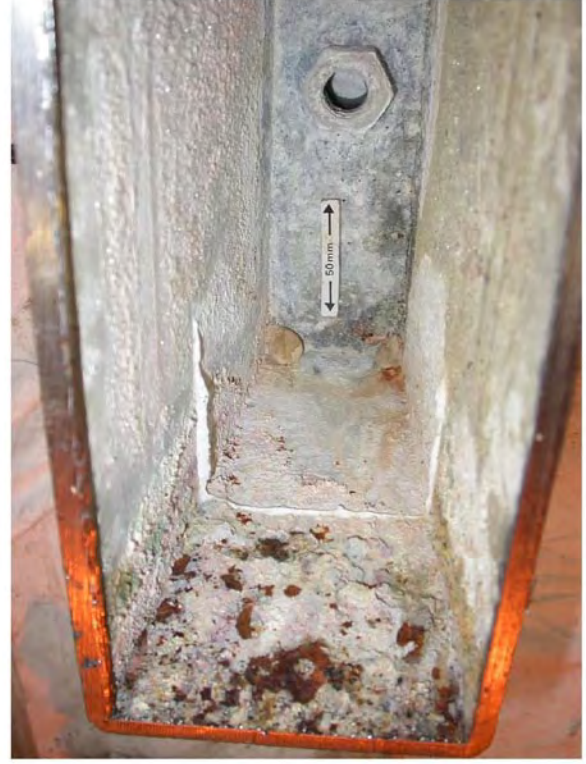
Figure 56: Detail of the internal water mark and long standing corrosion which had exposed areas of the steel substrate.
