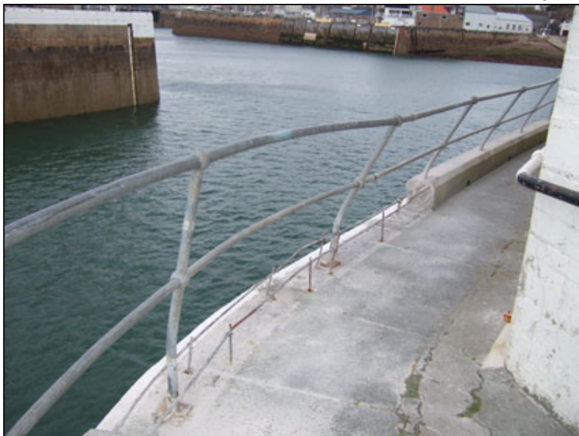
Damage to Victoria Pier head
