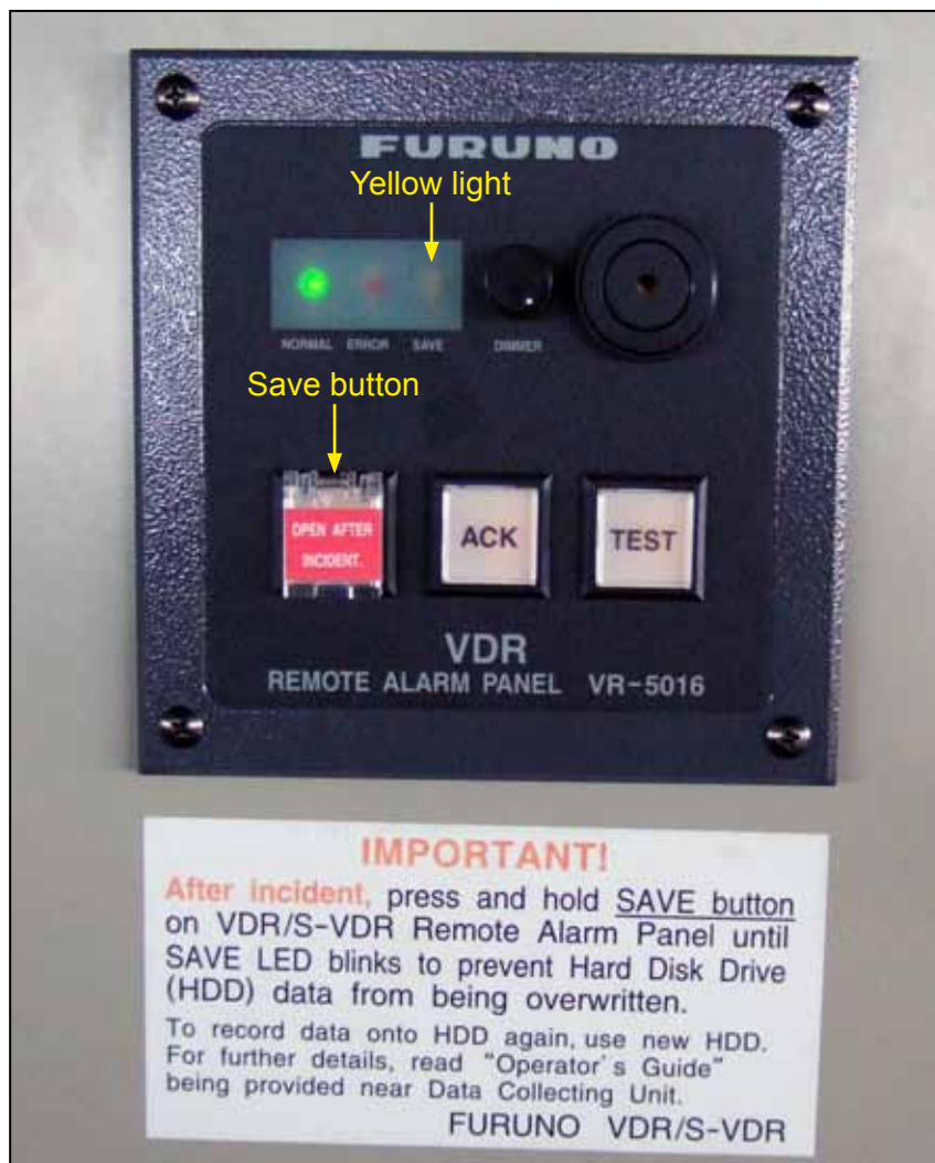
VDR - Remote alarm panel showing 'save' button
