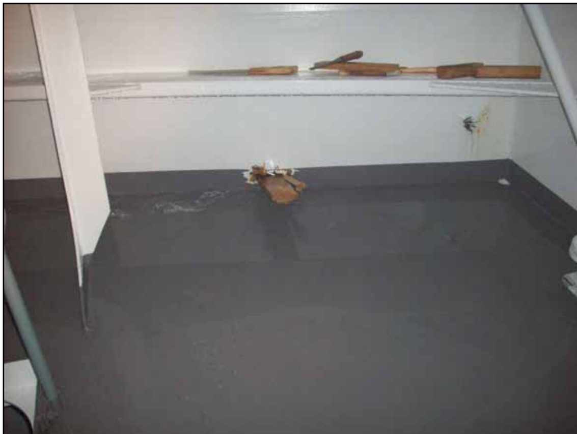
Example of bow thruster room damage control measures
