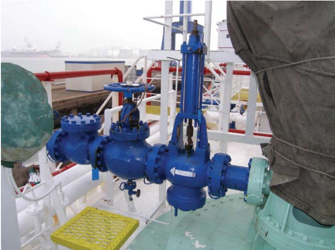
Sampling point and ESD valve
