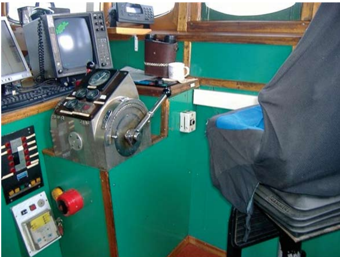
Operating panel at master's seat, looking to port
