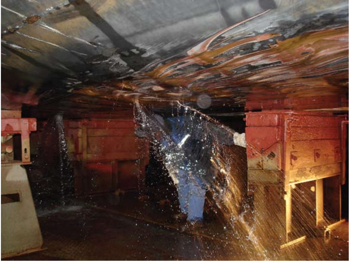
Damage below the waterline
