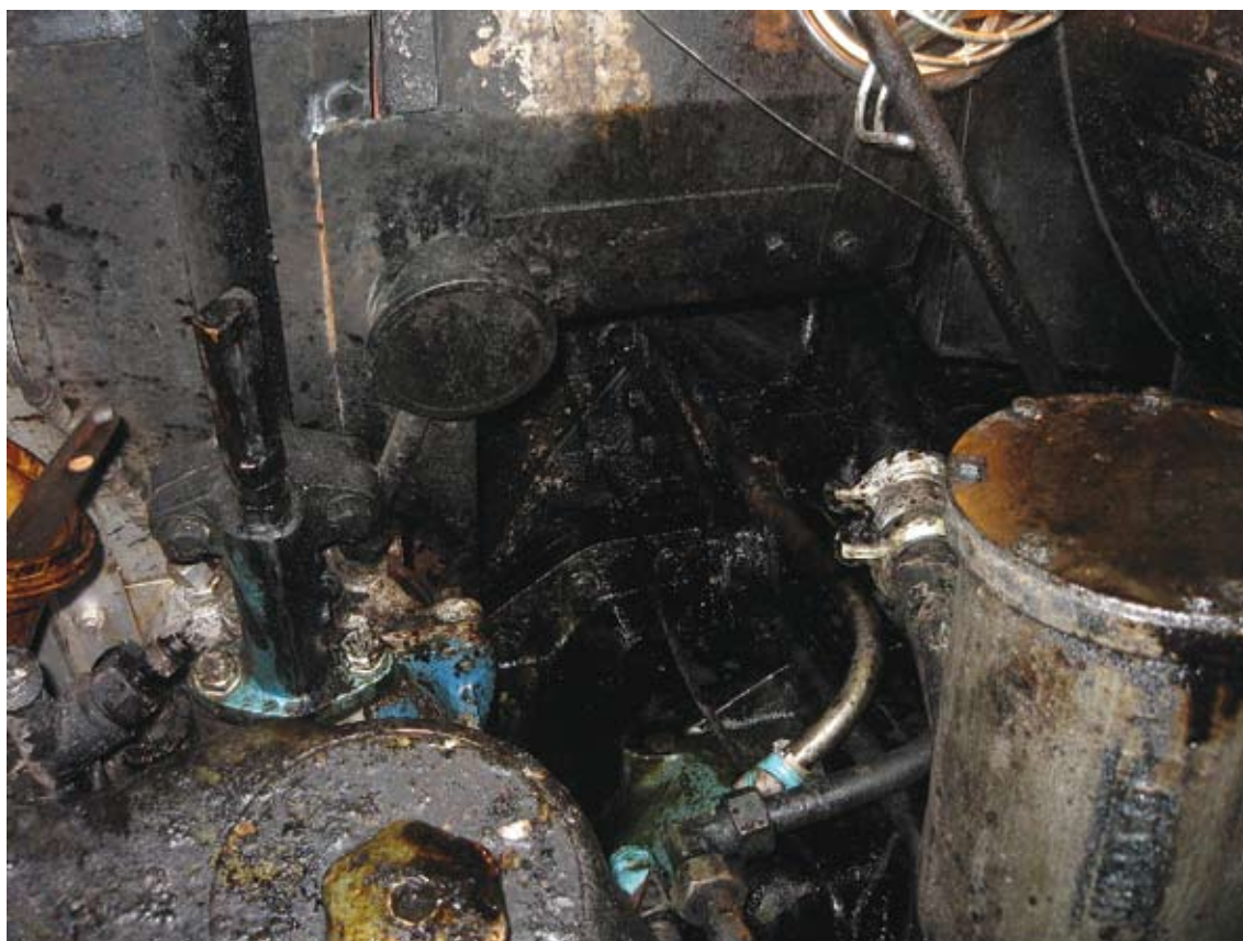
Figure 1 – Burst fuel pipe
