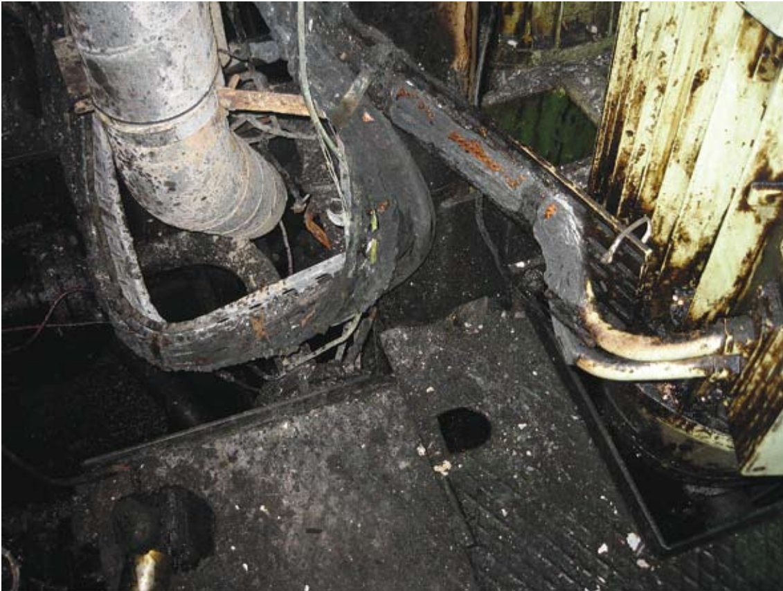
Figure 2 – One metre from the start of the fire
