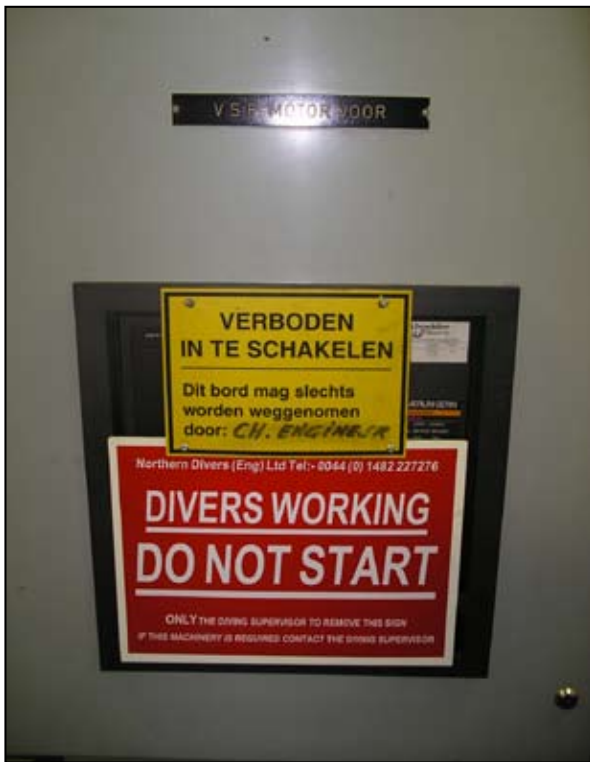
Warning sign on VSP switchboard
