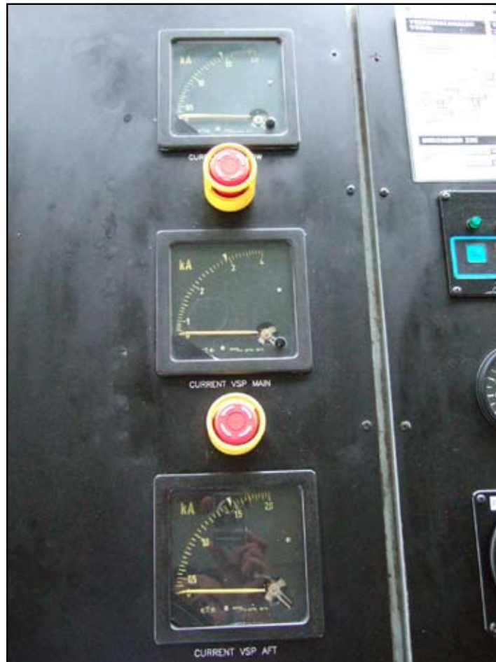
Ammeters on bridge control panel
