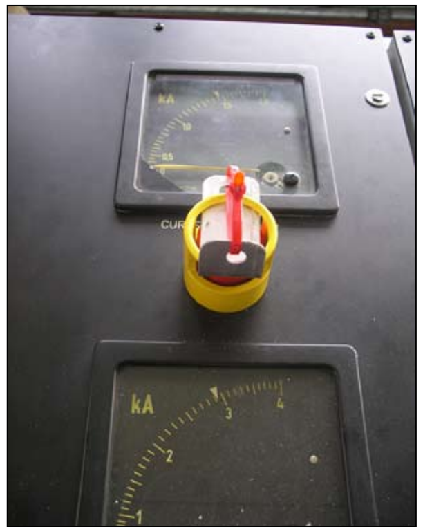
Emergency stops on bridge - measures to isolate motors from activation
