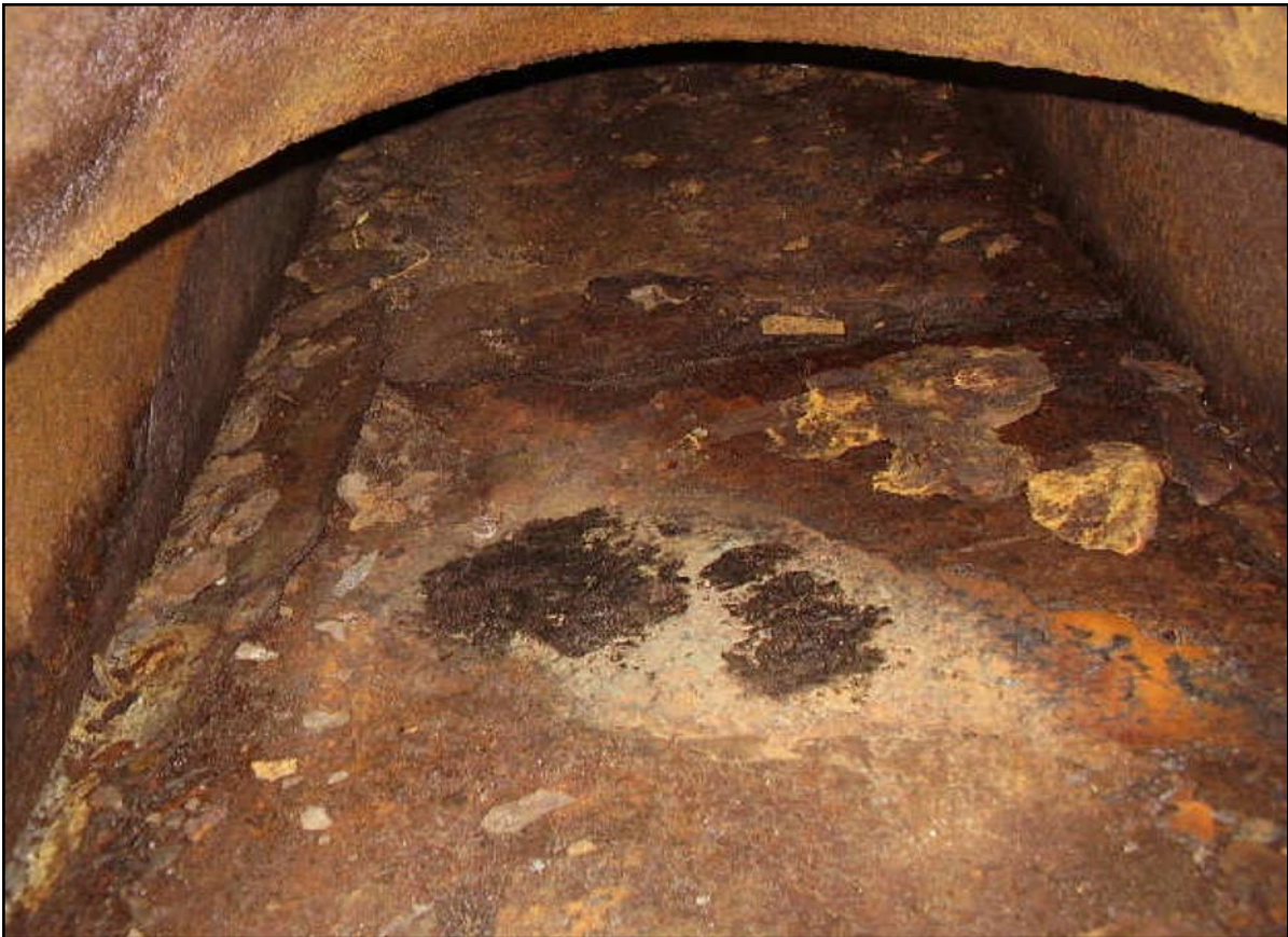
Damage to ventilation duct
