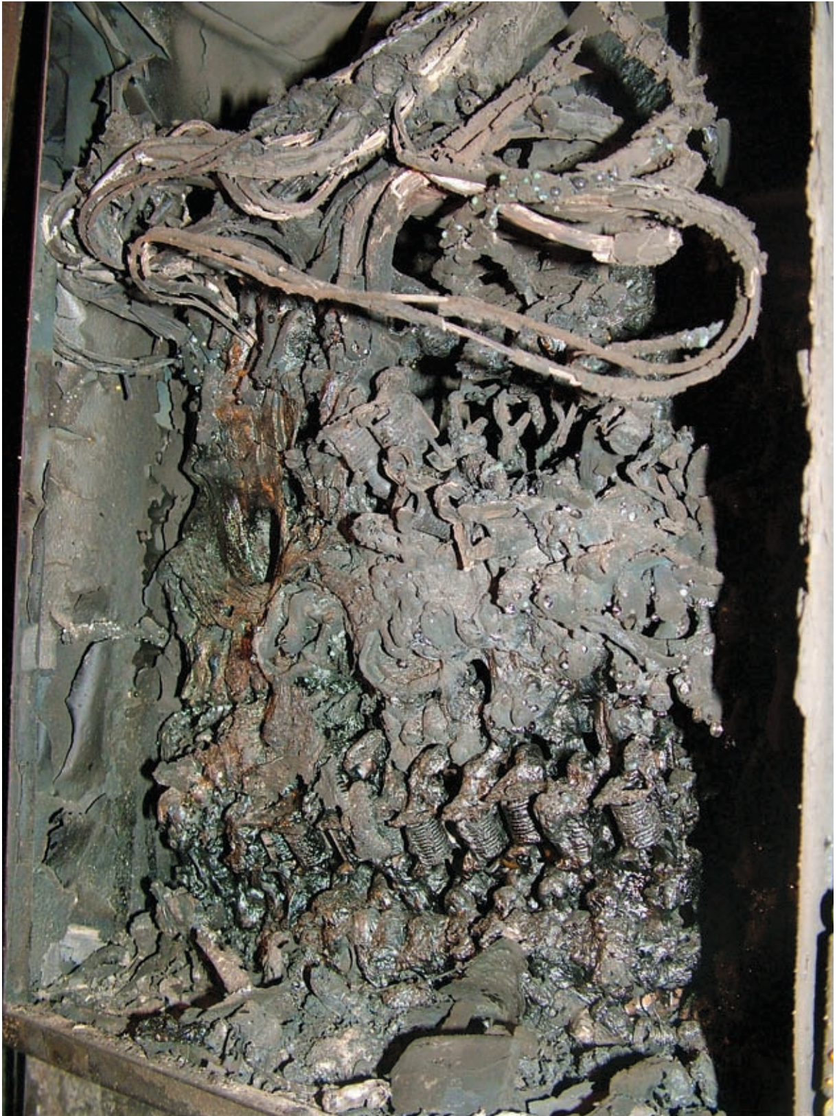
Figure 5: Damage to the 220v distribution panel
