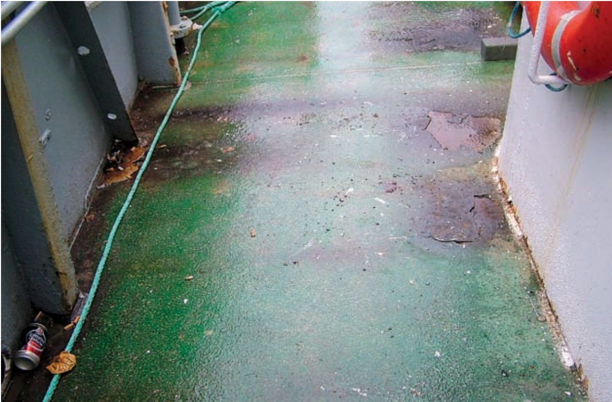
Figure 2: Blistering of the paint on the main deck
