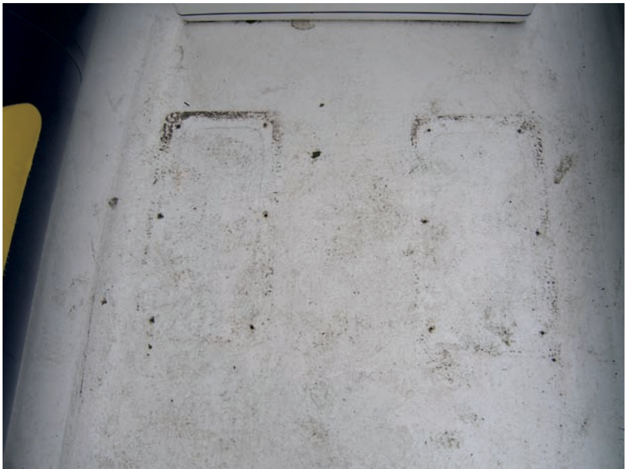
Vessel's deck showing outline of consoles – note lack of deck preparation and adhesive
