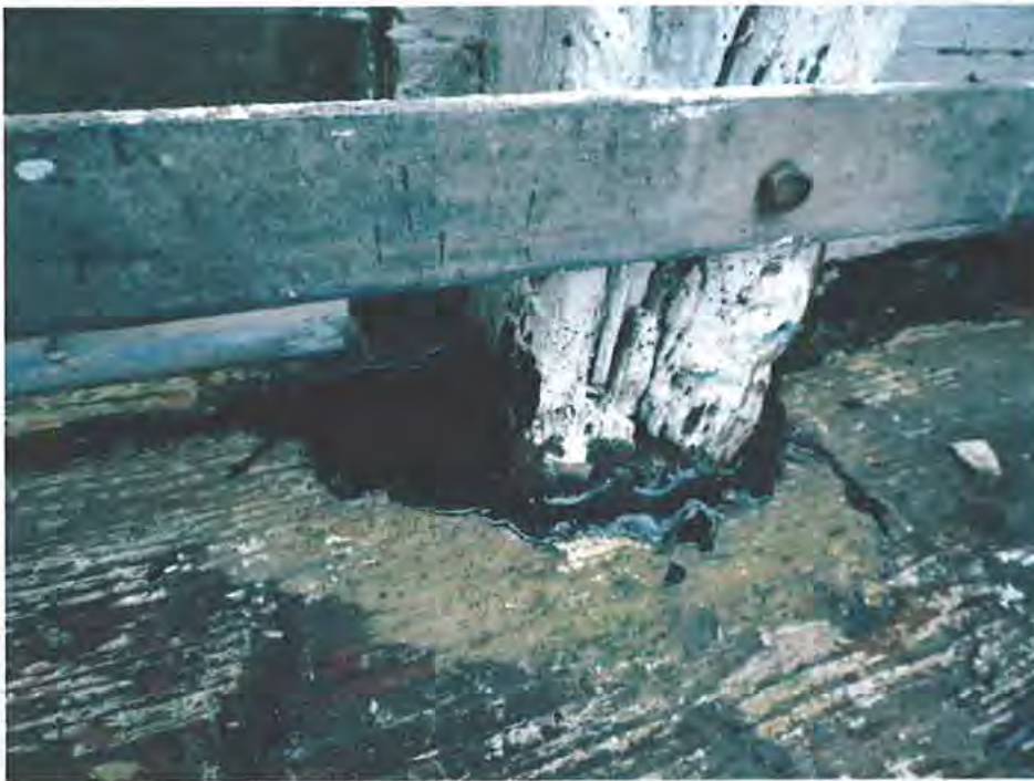
Fig 2. This shows a bulwark stanchion as it passes through the margin plan of the deck. Poured-in melted pitch has been recently applied.
