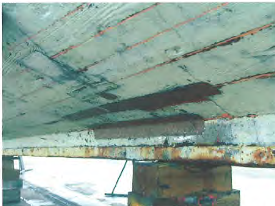
Fig 4 This shows new tingles being fitted to the garboard seam and the seam above. A small square tingle is fitted in the middle of plank No 2 another across the seam immediately above. Above this a larger rectangular tingle is fitted spanning plank No. 4 and the adjacent seams. The fact that all these are in a line across the vessel indicates to me that movement and leakage is occurring here.
