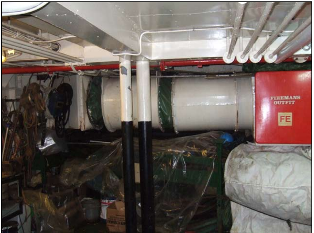
Forward store - port cargo ventilation trunking
