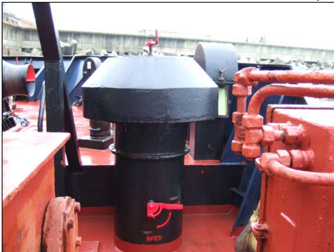
Starboard forward cargo mushroom ventilator and fire damper
