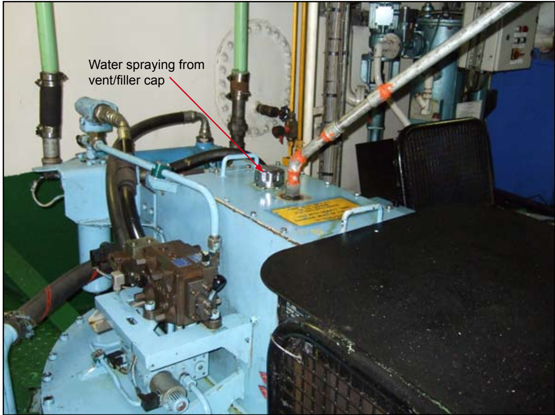
Photograph showing position of water ingress
