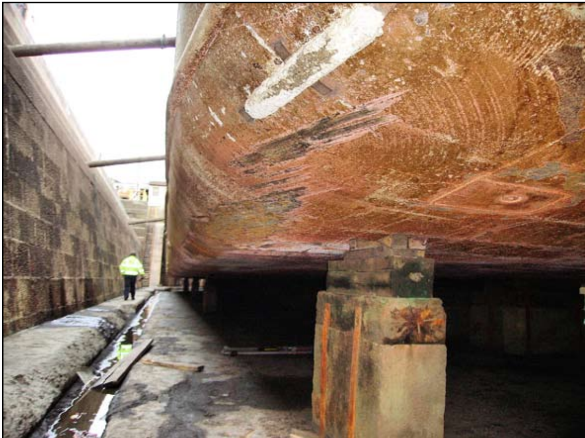
Paint damage to the underside of the hull on the vessel's port side
