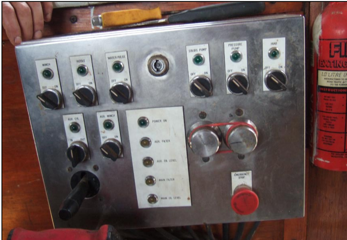
Hydraulic Control Panel
