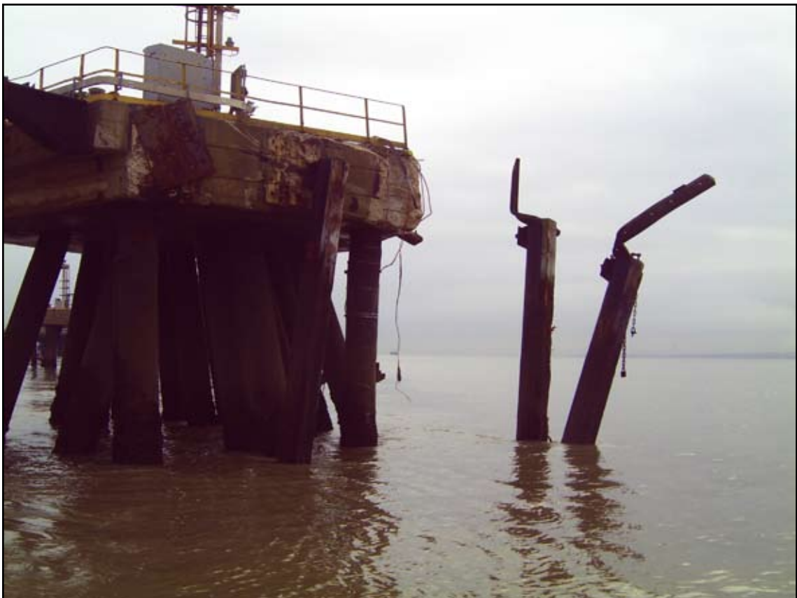
Damage to MD 41 mooring structure
