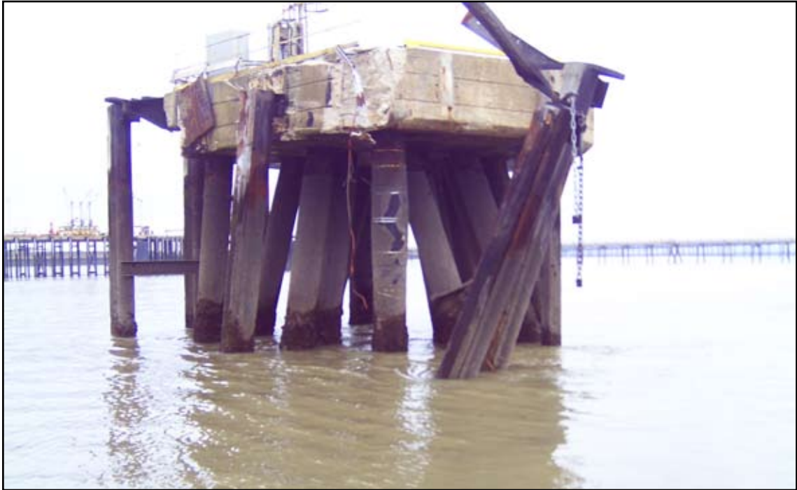
Damage to MD 41 mooring structure
