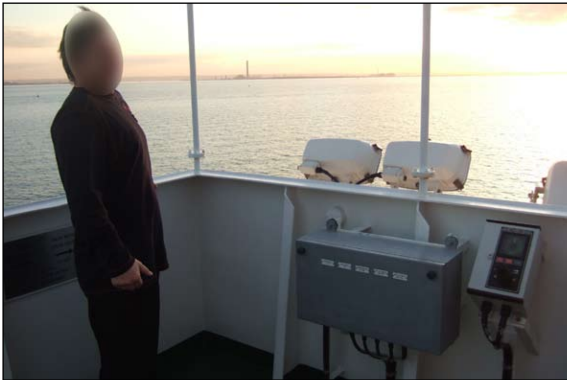
Bridge wing and bow thruster control
