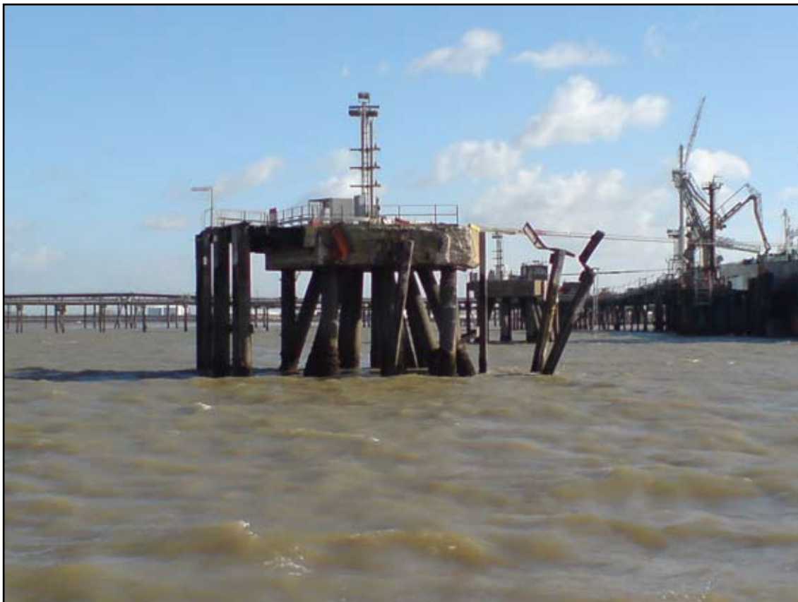
Damage to MD 41 mooring structure and stern lines leading to Thornbury
