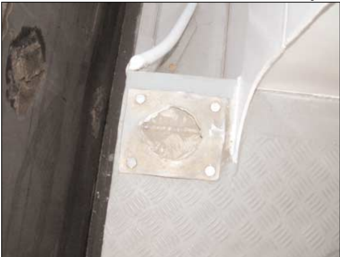
Failed Mk I bollard
