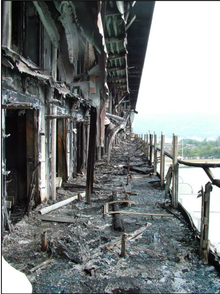
Melted aluminium structure
