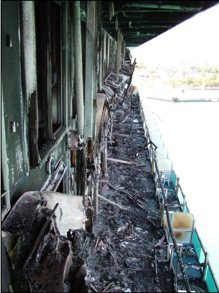
Damage to balconies
