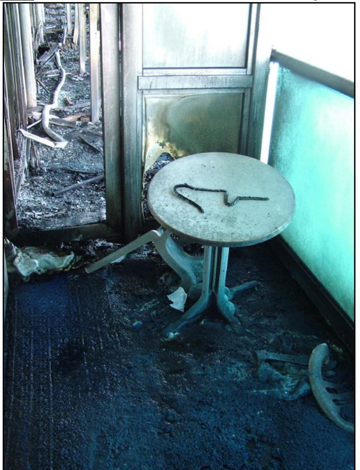
Partially melted balcony furniture
