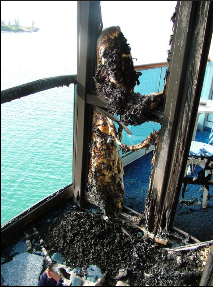
Melted polycarbonate partition
