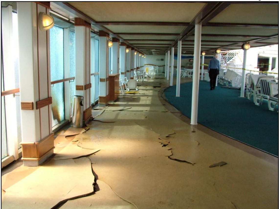
Damage to deck 14
