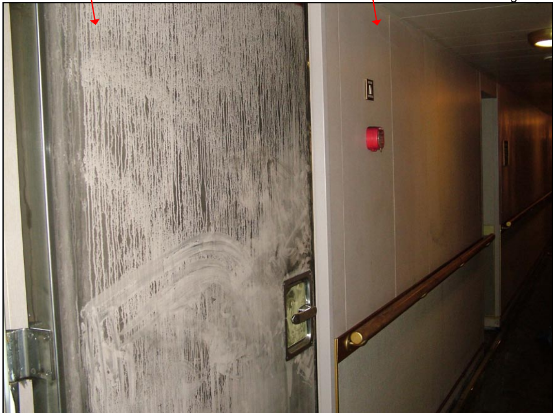
'A' class fire door between zones 3 and 4 on deck 12, port side
