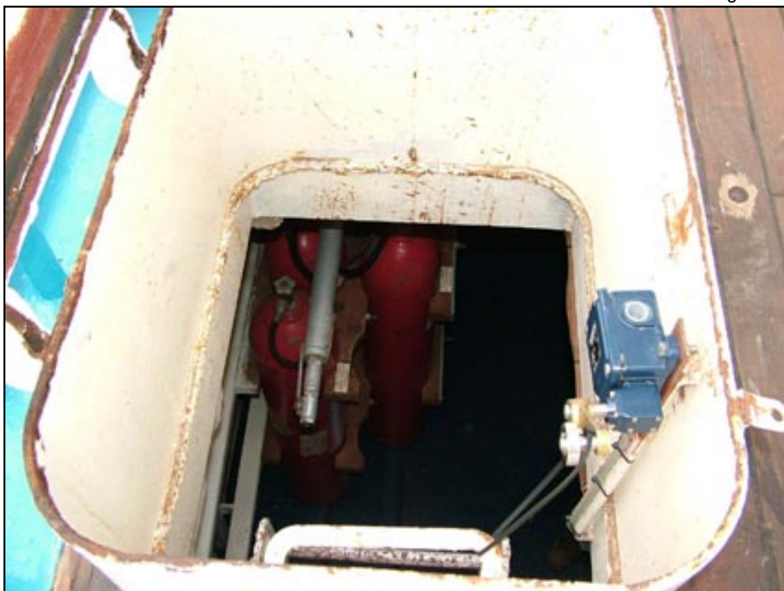
CO2 space hatch and access ladder
