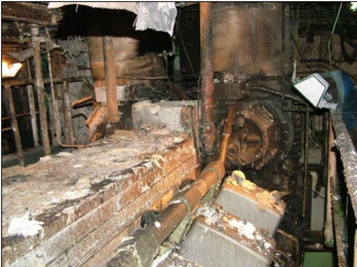
Fire damaged turbo chargers
