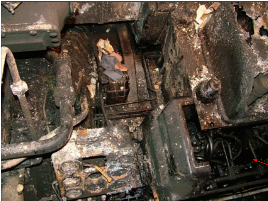
Forward end of hotbox of starboard engine
