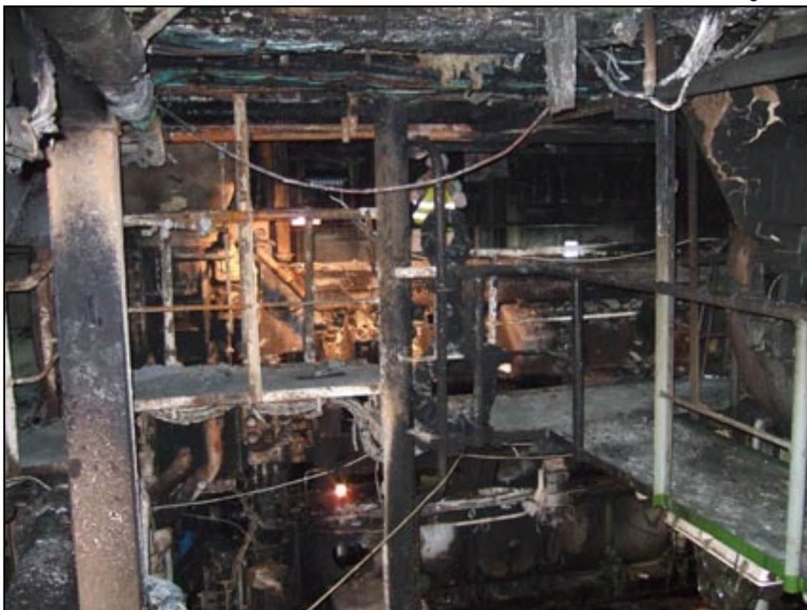
Damaged upper areas
