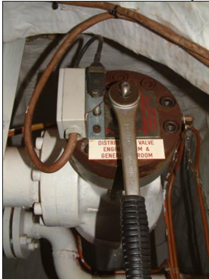
Engine room distribution valve with manual handle attached
