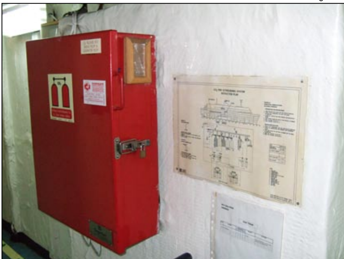
Remote CO2 release station for engine room
