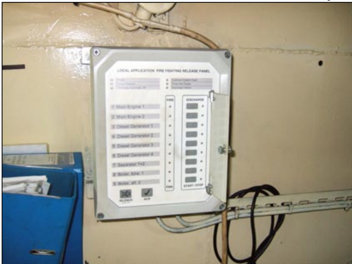
Low fog control panel
