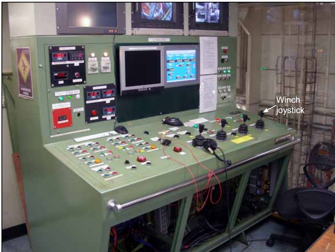
Dive control room
