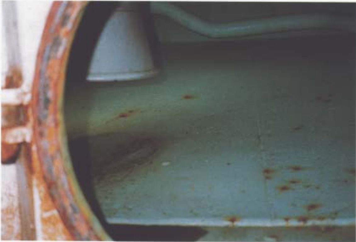
End of fish suction pipe (elephant's foot) in RSW tank
