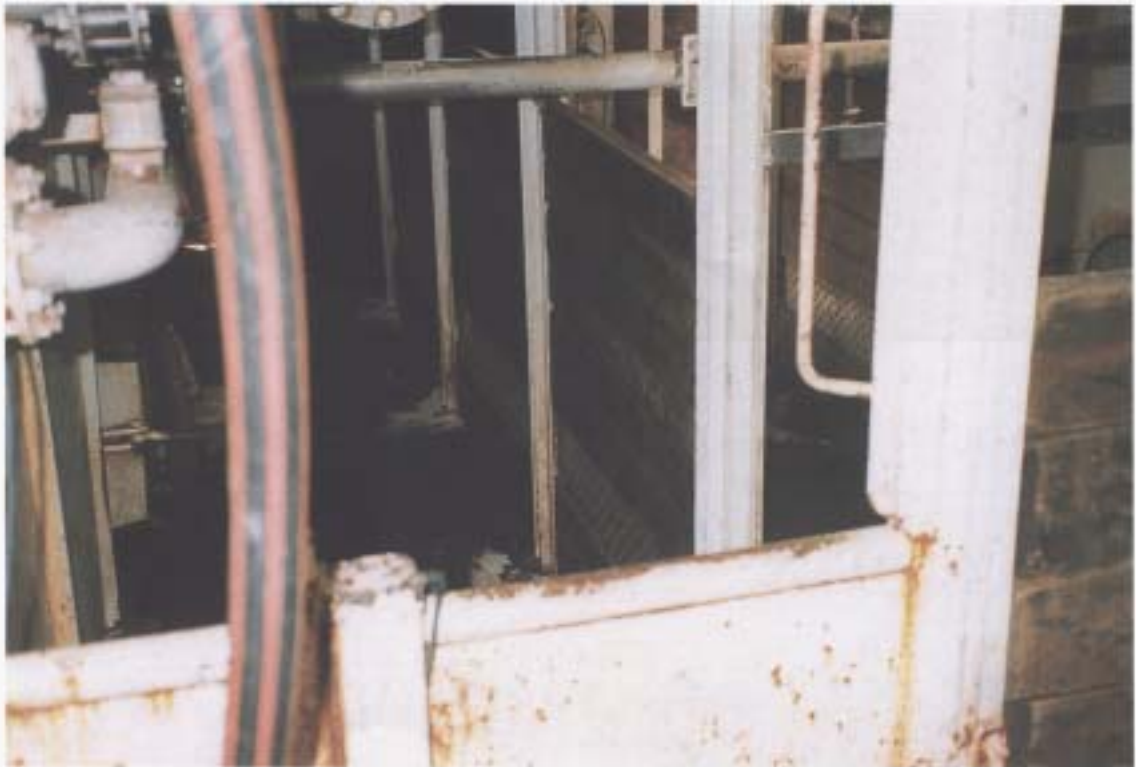
Starboard side of ramp deck in area of accident
