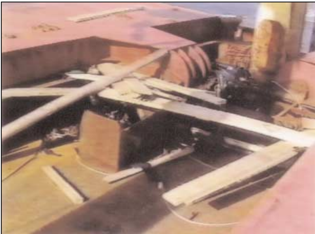
Photograph showing space between hatch hold covers
