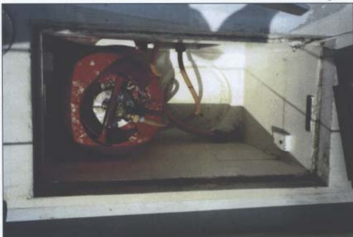
Interior of ready-use gas bottle locker with one bottle and the bottles' securing arrangement removed
