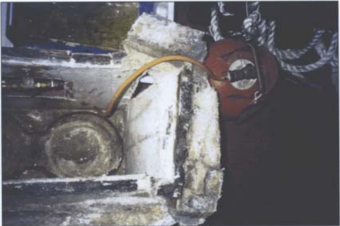
Ready-use gas bottle locker moulding following accident
