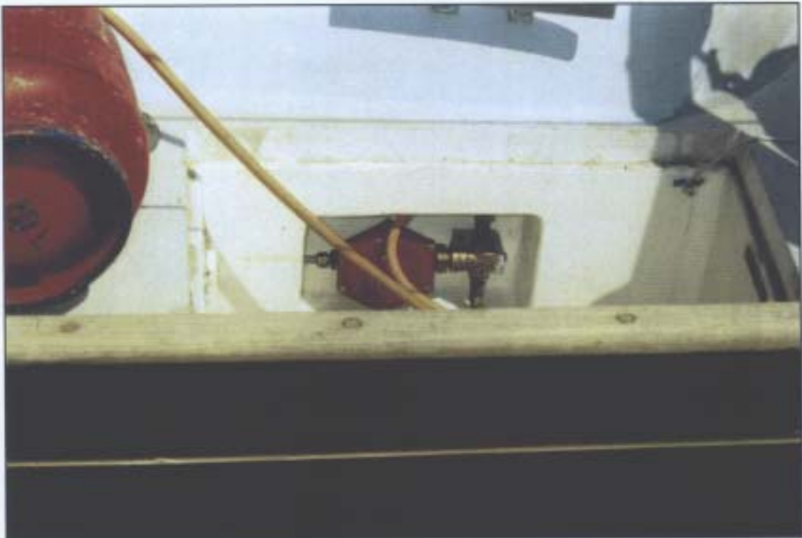
Moulded recess in ready-use gas locker accommodating 'T' piece wallblock and pressure regulator
