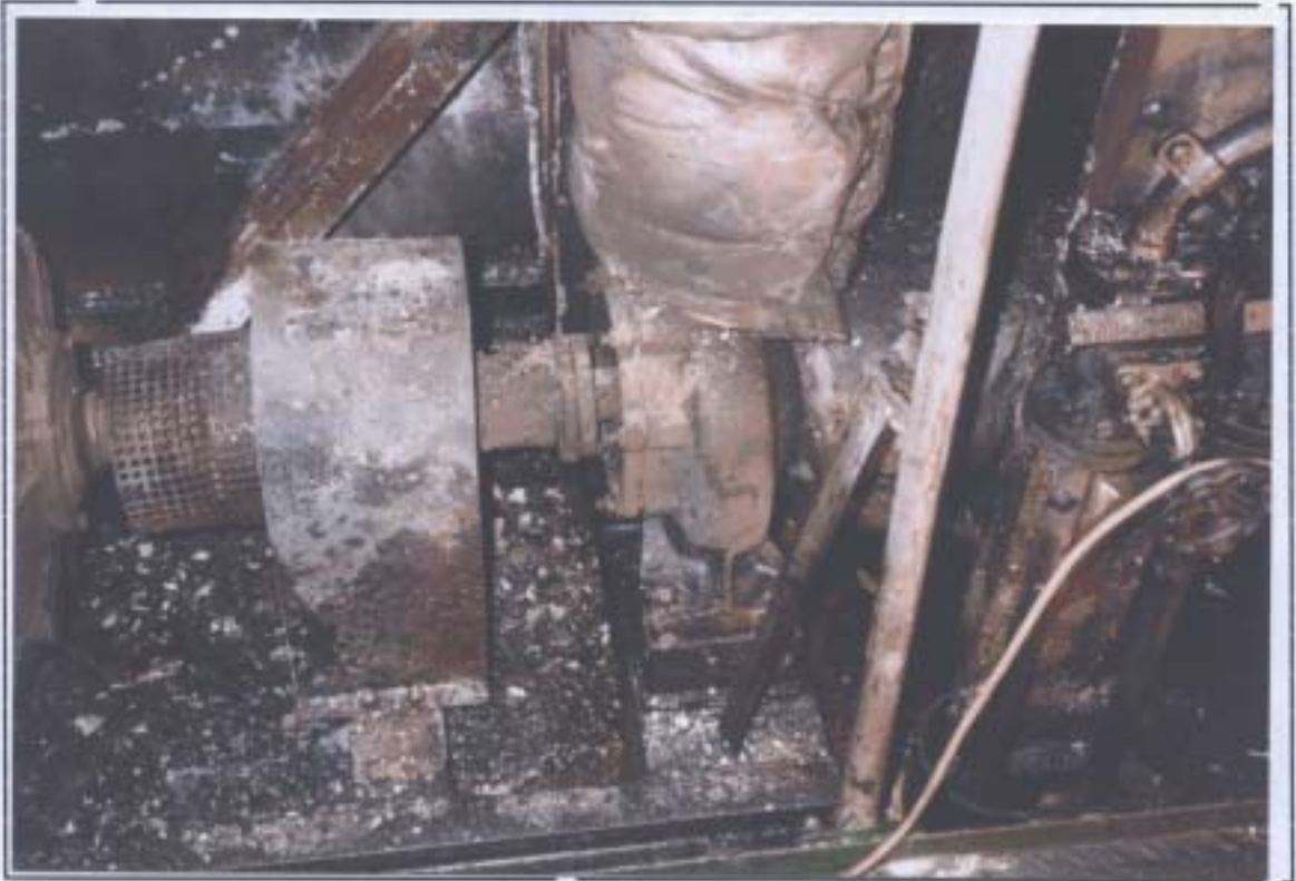
Fig 2 Close-up view of No 2 starboard thermal oil pump showing shrouded coupling and bearing bracket.
