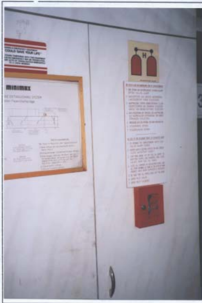
Fig 8 General view of Halon Control Station on deck 3. Note instructions and locked key box.
