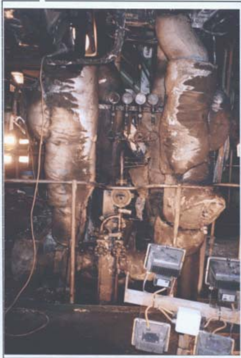
Fig 1 General view of No 2 Thermal Oil Pump. Return lines the right, discharge lines on the left.
