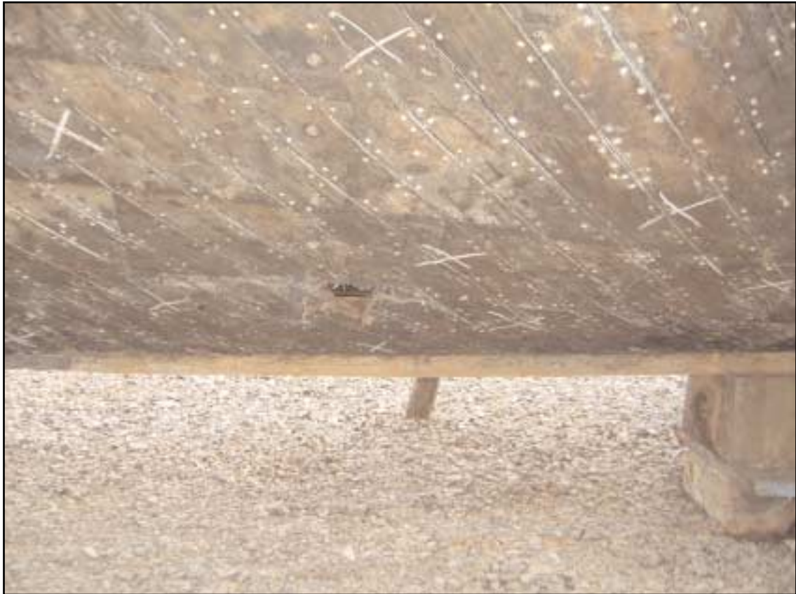
A hole in the port side of the hull in way of the bar/buffet space
